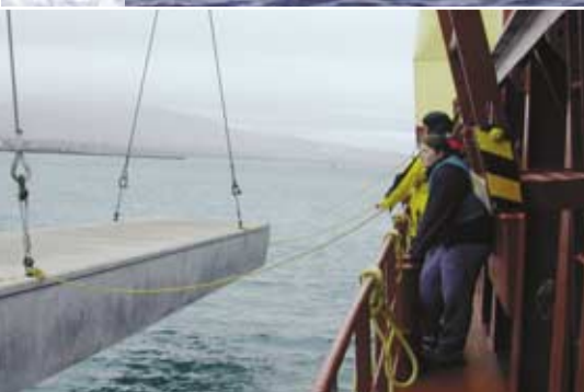
BELOW: An all concrete pontoon being lowered from the ship against the misty backdrop of Valentia Island.
